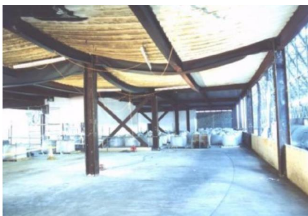
Figure 1-1: Deformation of steel beams under a test fire [1]
