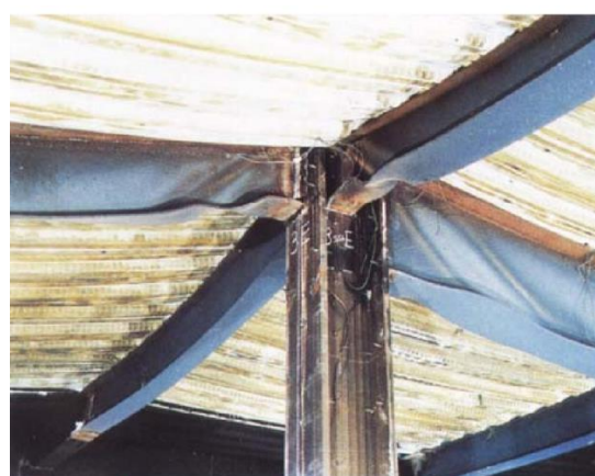
Figure 1-2: Deformation of beams near a column after a fire test [1]
