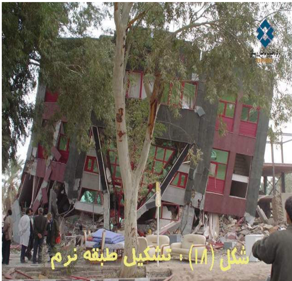
Fig. 1-1: Recently-constructed building collapsed from earthquake tremors in Bam, Iran (Courtesy of BHRC)
