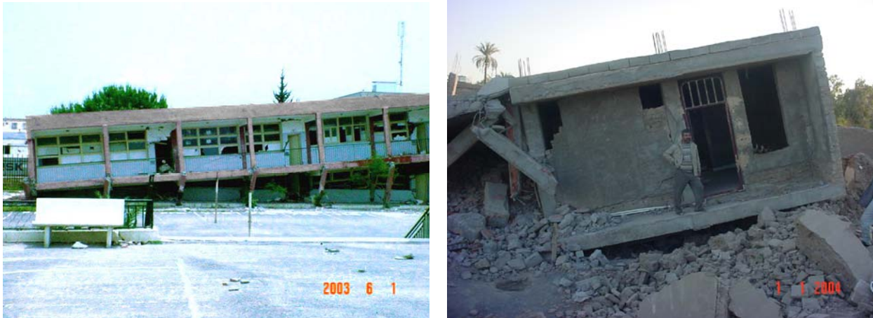
Figure 4-7: Soft-storey ground floor of a school, Boumerdes, Algeria [11], and of a house in Bam, Iran [Courtesy: Astan-Qods-Razavi]
