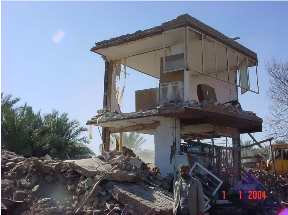
Figure 3-12: Damage to brick masonry buildings in earthquake, Iran [31]
