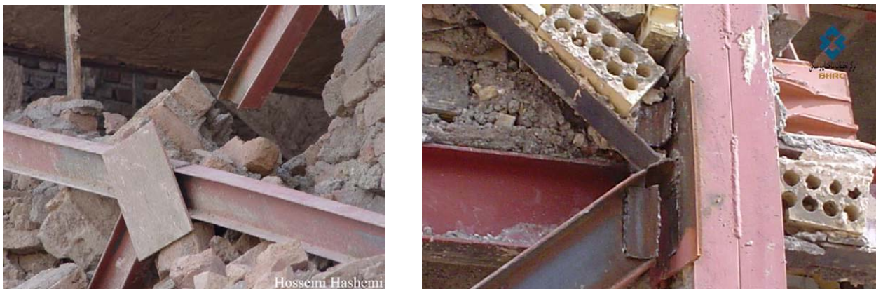
Figure 4-18: Poor quality of welding on site proved after earthquake in Bam, Iran [31]
