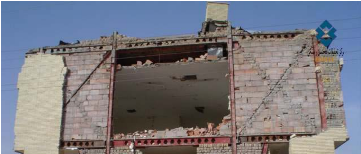
Figure 4-16: Good performance of small fields of infill walls in comparison with large fields during the earthquake in Bam, Iran [31]
