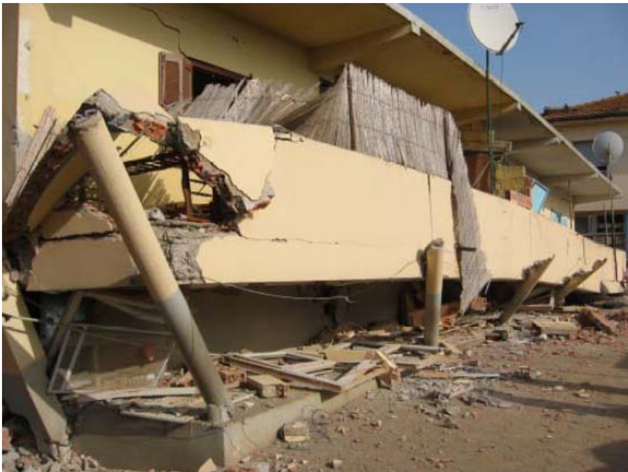
Figure 4-9: Elementary school collapsed because of insufficient lateral resisting system and soft-storey, Boumerdes, Algeria [11]
