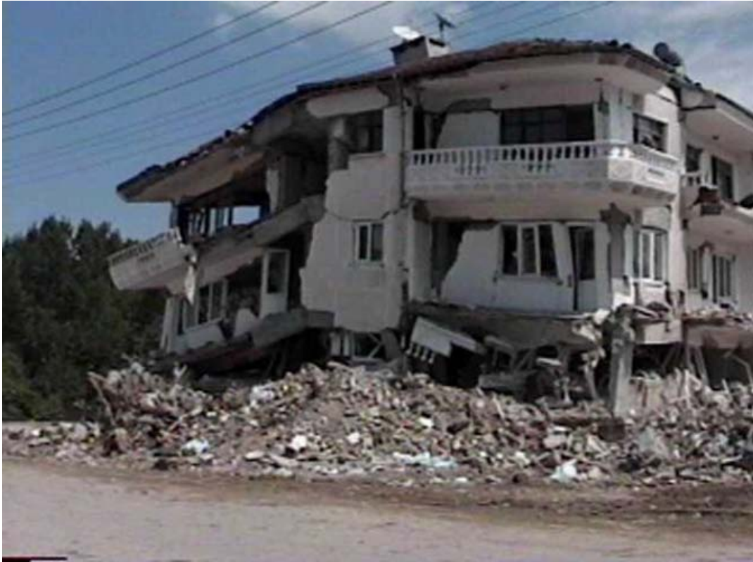
Figure 4-6: Collapse due to asymmetry in the plan, Yalova, Turkey [12]
