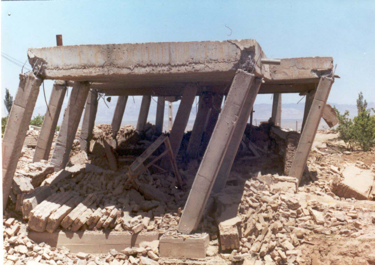
Figure 3-14: Damage to reinforced concrete buildings due to inadequate horizontal load resisting systems in Ardakul earthquake, Iran [31]
