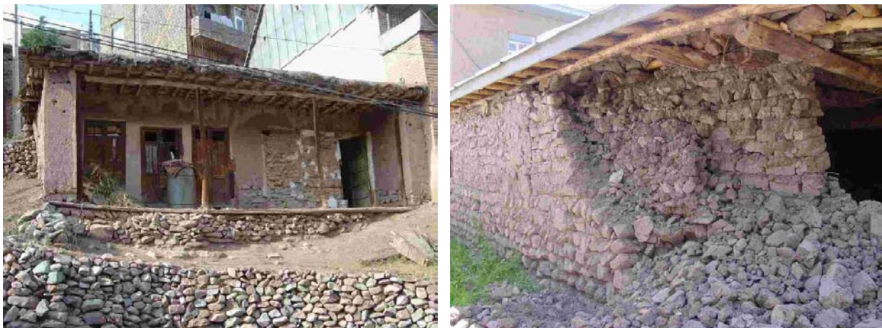
Figure 3-11: A typical stone building in Iran and a damage pattern in external walls during earthquake [9]
