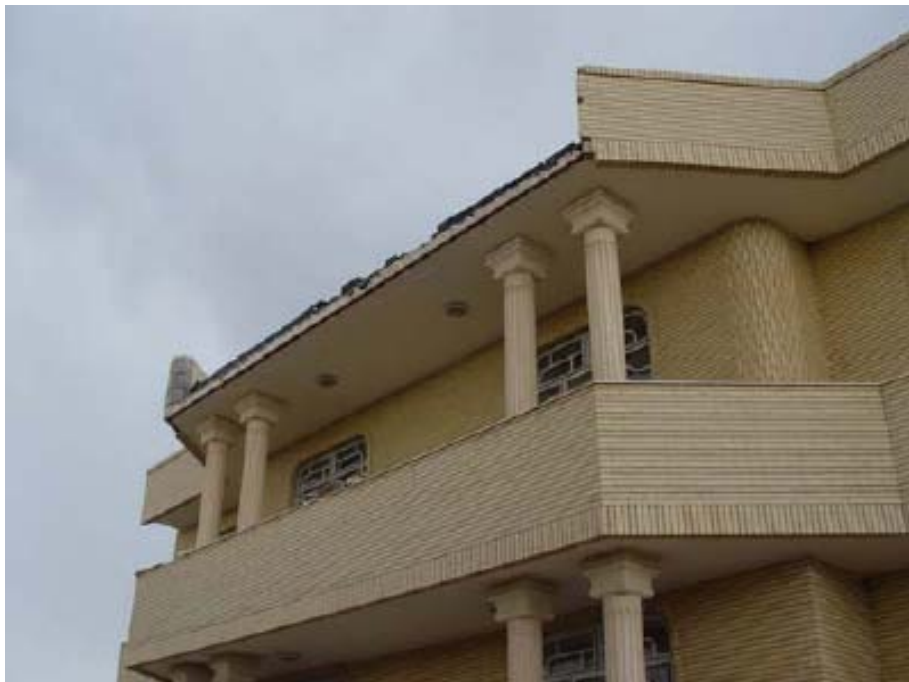
Figure 4-19: Damage due to the failure of facade after earthquake in Bam, Iran [31]
