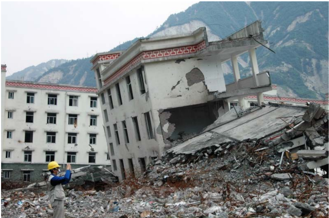
Figure 4-1: Collapse of a school building in Sichuan, China [13]
