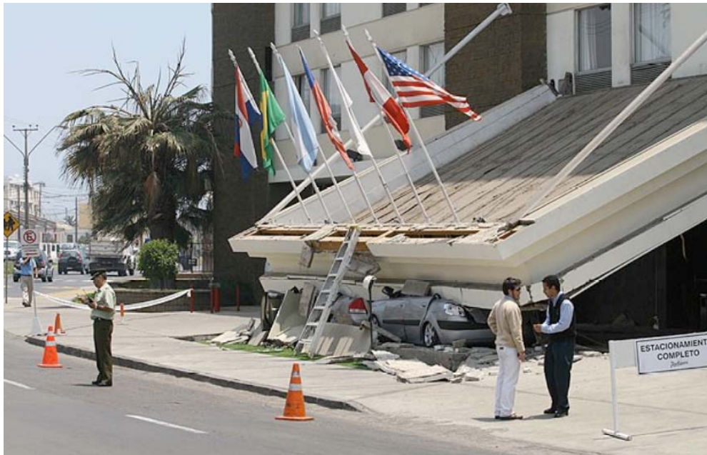
Figure 4-3: Roof collapse in the city of Antofagasta, Chile [15]
