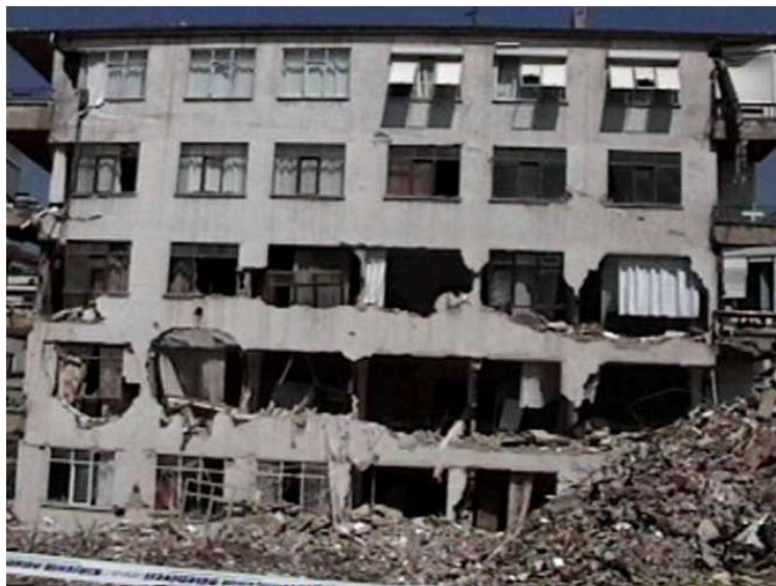
Figure 4-8: Collapse of a wall with large openings, Yalova, Turkey [12]
