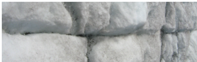
FIGURE 7.7: Picture of a crack that was observed during FT-0.0.
