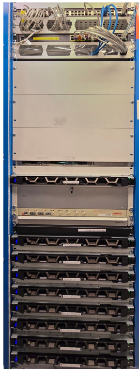
Figure A.2: DCS rack in SDX1 Level 2 with deployed EMP test crate (below the three large empty white cover panels)
