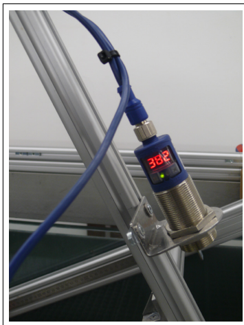
(A) Ultrasonic displacement sensor for accurate measurement of water levels
