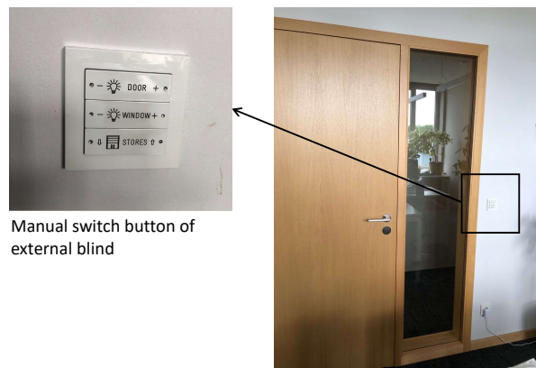
Figure 5.7: The manual switch of the external blind 5
